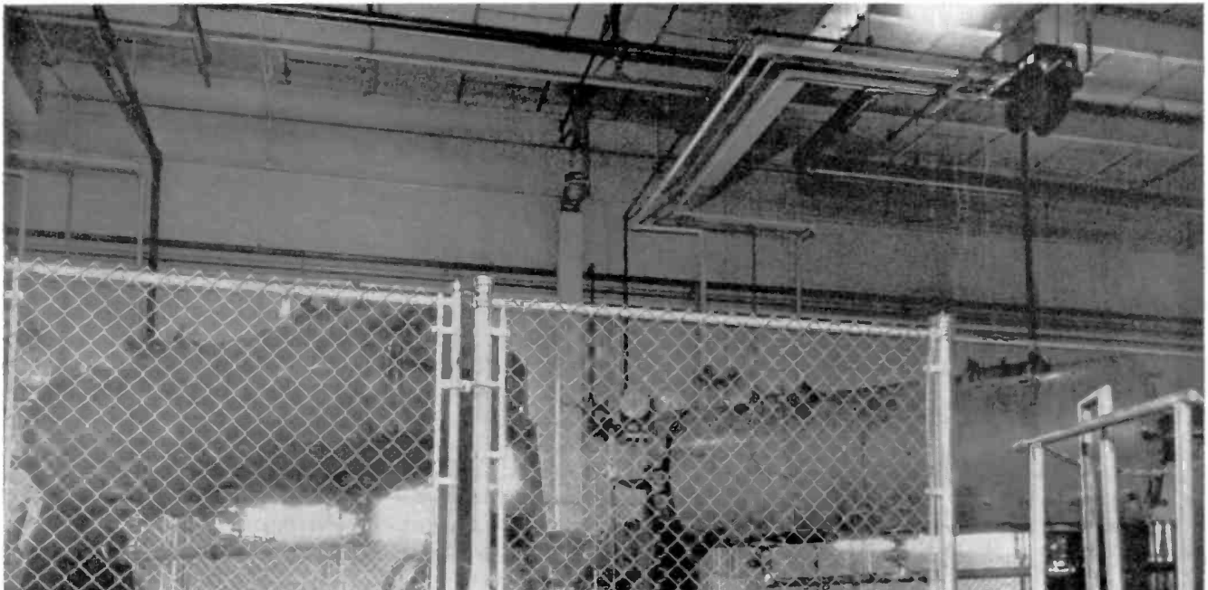
Last step before coating is the milling of the oxide and binder ingredients to produce a homogenous mass without lumps. These ball mills are installed in the new plant of the Reeves Soundcraft Company in Danbury, Connecticut. Like the previous steps in the manufacture of tape, this milling is also a rather critical process.
