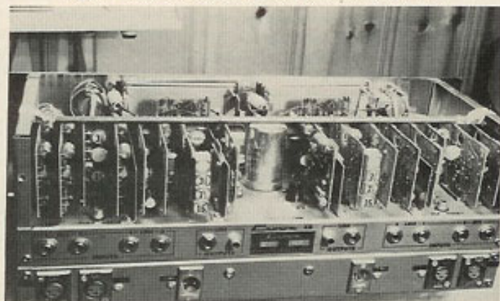
Fig. 12—Back view of complete electronics chassis.
